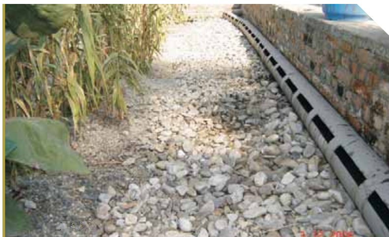
Slotted pipe inlet
