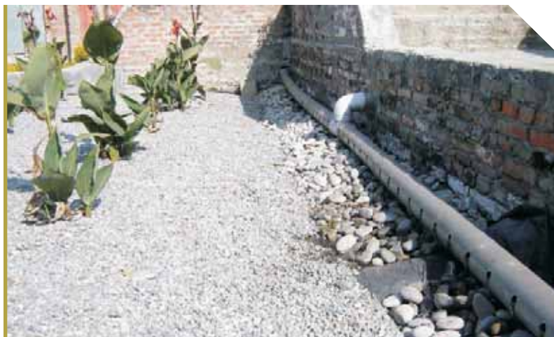
Perforated pipe inlet
