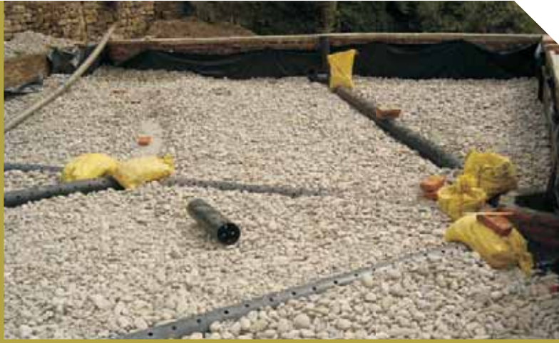
Installation of collection network and filling of substrate (drainage layer) in vertical flow CW
