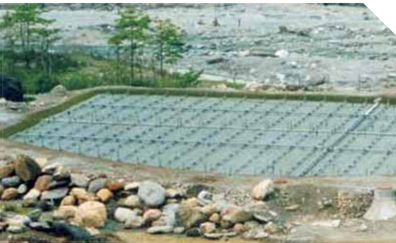
Vertical flow constructed wetland (Shrestha R.R.)
